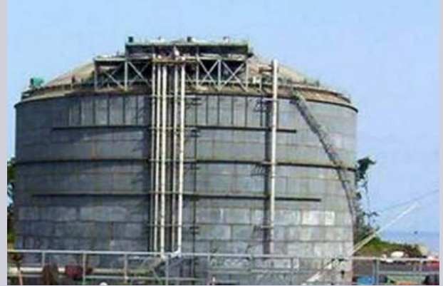
Barzan Gas Project, Ras Laffan Industrial City
